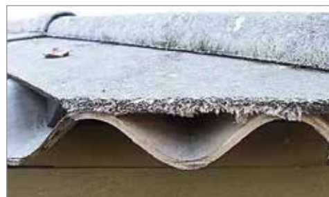
Asbestos-containing roofing felt
